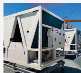
Hungarian Cédrus Liget. A complex facility including apartments, offices and commercial units. Szeged, Hungary. ECOi-W, ECOi and ERV.
